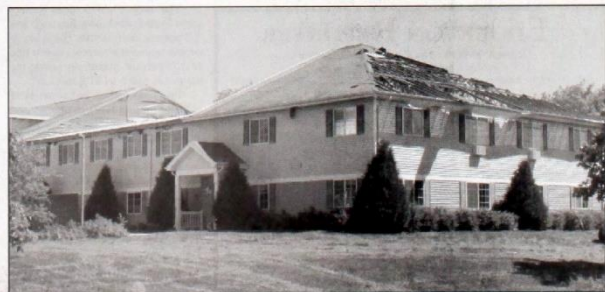
SERVPRO began the main restoration project on the Edgewood Glen Senior Apartments on Monday, beginning with the tearing down and rebuilding of about 80 percent of the roof. Edgewood Glen was set ablaze in May after being struck by lightning. (Edgerton Reporter photo/Michael Gouvion)
